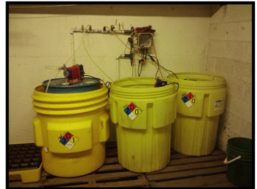
Dual containment drums in the UNT System Building basement.
